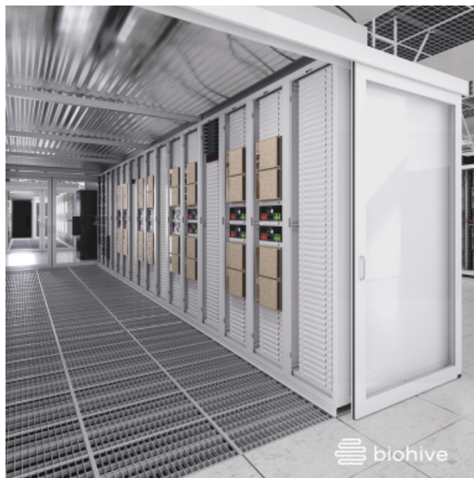
Figure 20. We believe BioHive-1 is one of the most powerful supercomputers dedicated wholly to drug discovery for a single company. This rendering shows what BioHive-1 might look like when installed, expected to be in early 2021. The supercomputer further expands our capability to rapidly improve ML models.
